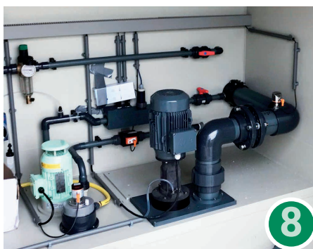
Station de pompage
